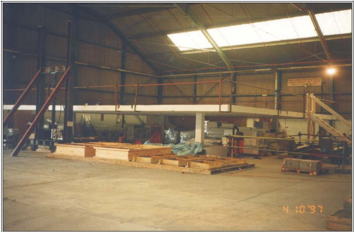
Figure 4.58: Structure B (Configuration 1) - General View of Structure B in its Bare Condition.
