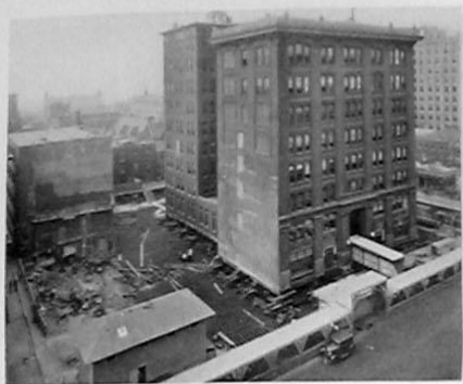
FIGURE 4. As the building appeared on October 14 ready for the move to start.
