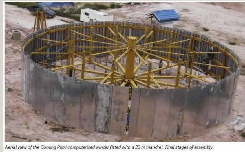
Aerial view of the Gunung Putri computerised winder fitted with a 20 m mandrel. Final stages of assembly.
