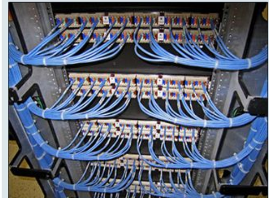
Network cable is used to connect computers and devices to a network.
