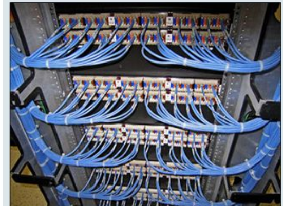
Network cable is used to connect computers and devices to a network.
