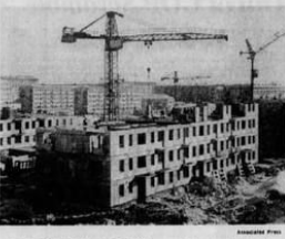
THE CONSTRUCTION CRANE is a symbol of activity in the Soviet Union. Here, new apartment buildings are going up in a Moscow suburb. Says one U.S. expert: "The Soviet Union can now produce a four-room apartment for $1000 to $1500 that would cost $10,000 in the United States."
