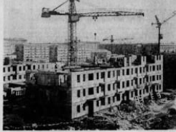
THE CONSTRUCTION CRANE is a symbol of activity in the Soviet Union. Here new apartment buildings are going up in a Moscow suburb. Says one U.S. expert: "The Soviet Union can now produce a four-room apartment for $3,000 to $3,500 that would cost $10,000 in the United States." The technique: mass-production.
