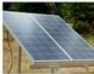
The billboard has 10 solar panels with each panel generating 100 watts of power.
