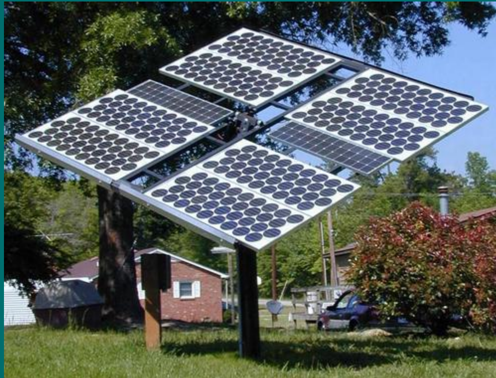
Solar electricity generation
