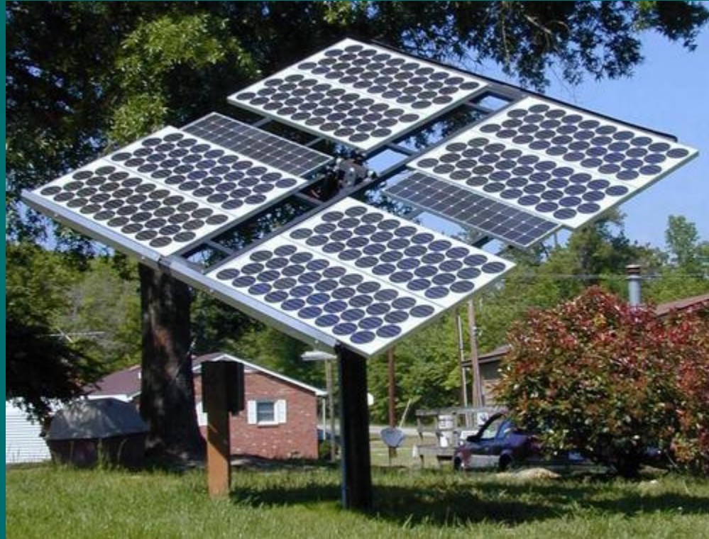
Solar electricity generation
