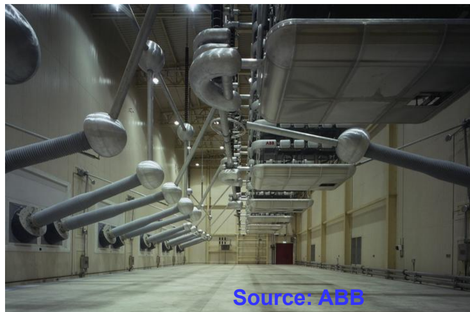
Thyristor valve hall
