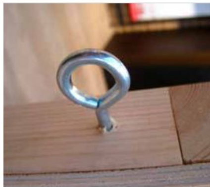
Screw in the eyebolts to the top corners of the wood panels
