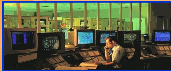
Head Office Remote Monitoring
