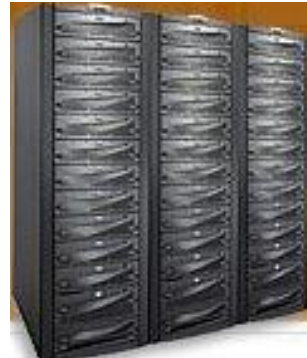
EMC CLARiiON and DMX Storage Array
