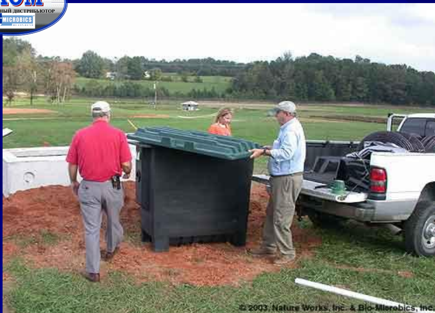
© 2003, Nature Works, Inc. & Bio-Microbics, Inc.
