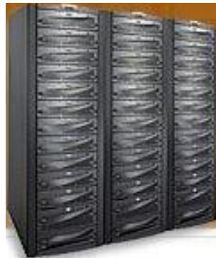
EMC CLARiiON and DMX Storage Array
