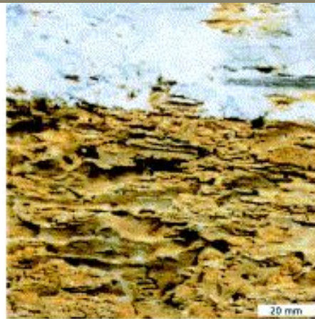
thick layers of limewash on damaged wood
