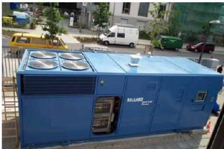
250kW Alstom Ballard Fuel Cell Power Plant, installed with Bewag AG in Berlin, Germany. Source: Ballard
