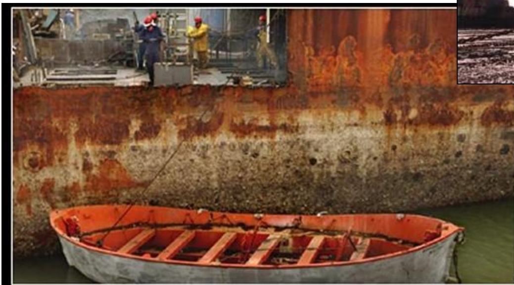
Workers cut away sections of the hull of a ship for scrap metal
